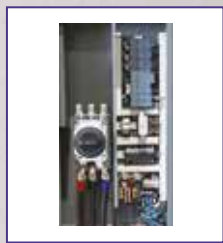
Control panel and Circuit breaker
